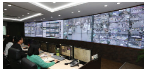
Integrated CCTV Control Center for Jongro-gu district, Seoul
